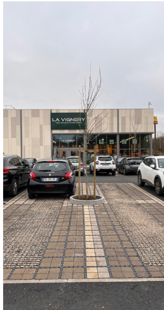
The renovation of the car park at Portes de Taverny, with water permeable pavers
