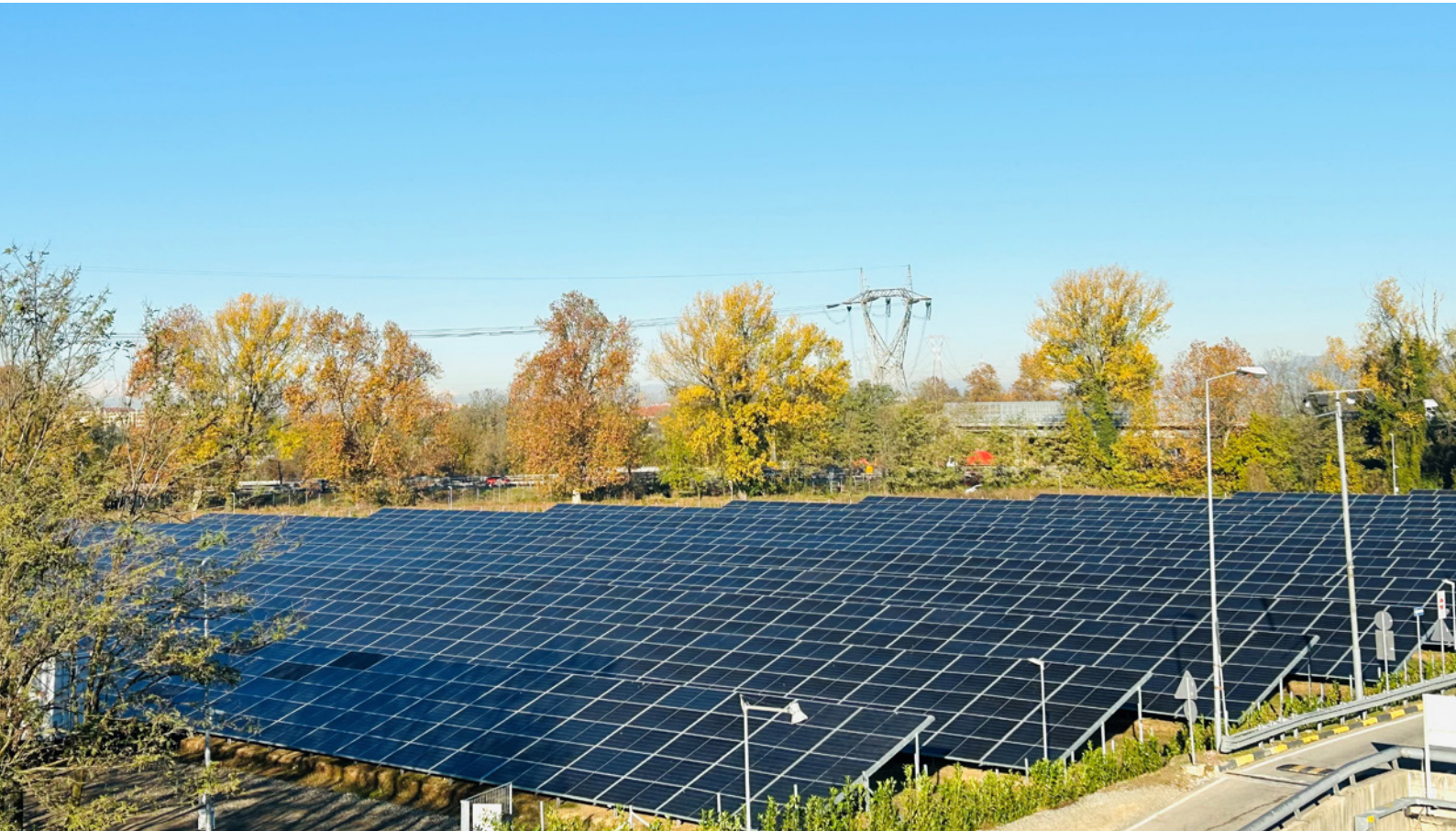
Solar panels at Carosello Shopping Centre
